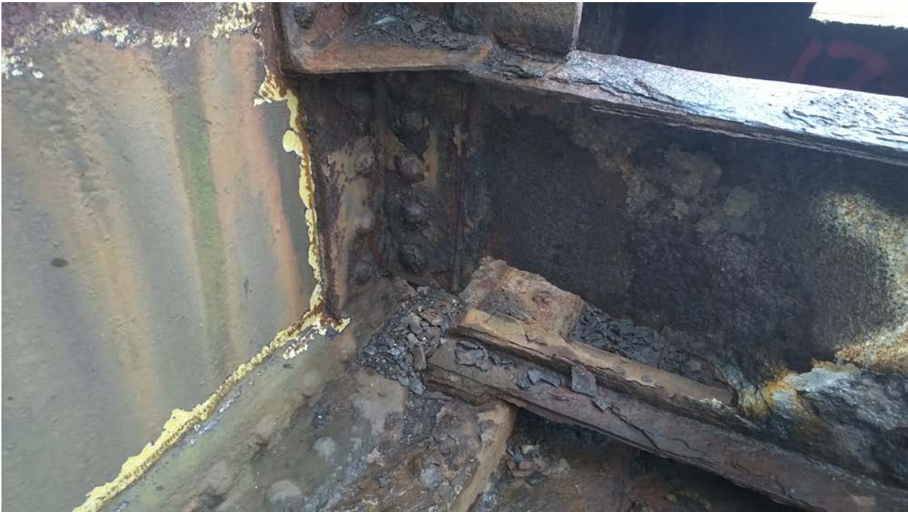
Photo 1 - Corroded cross beam
