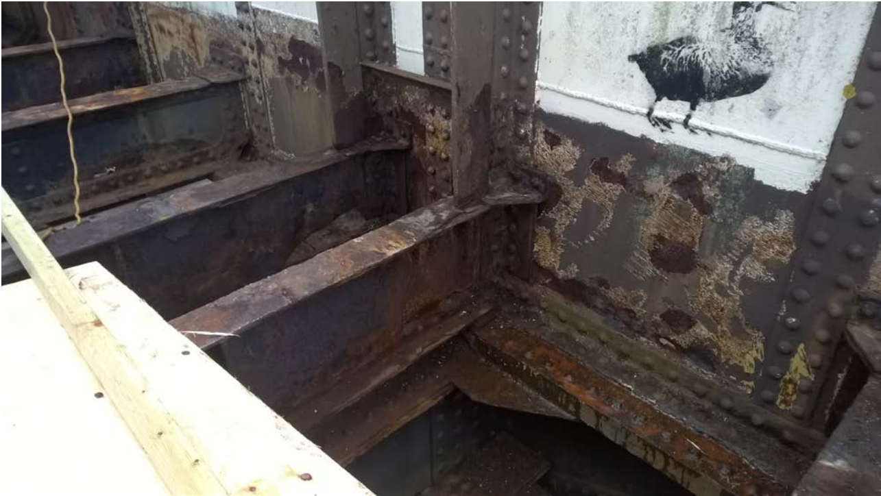
Photo 2 - Widespread corrosion below road surface level
