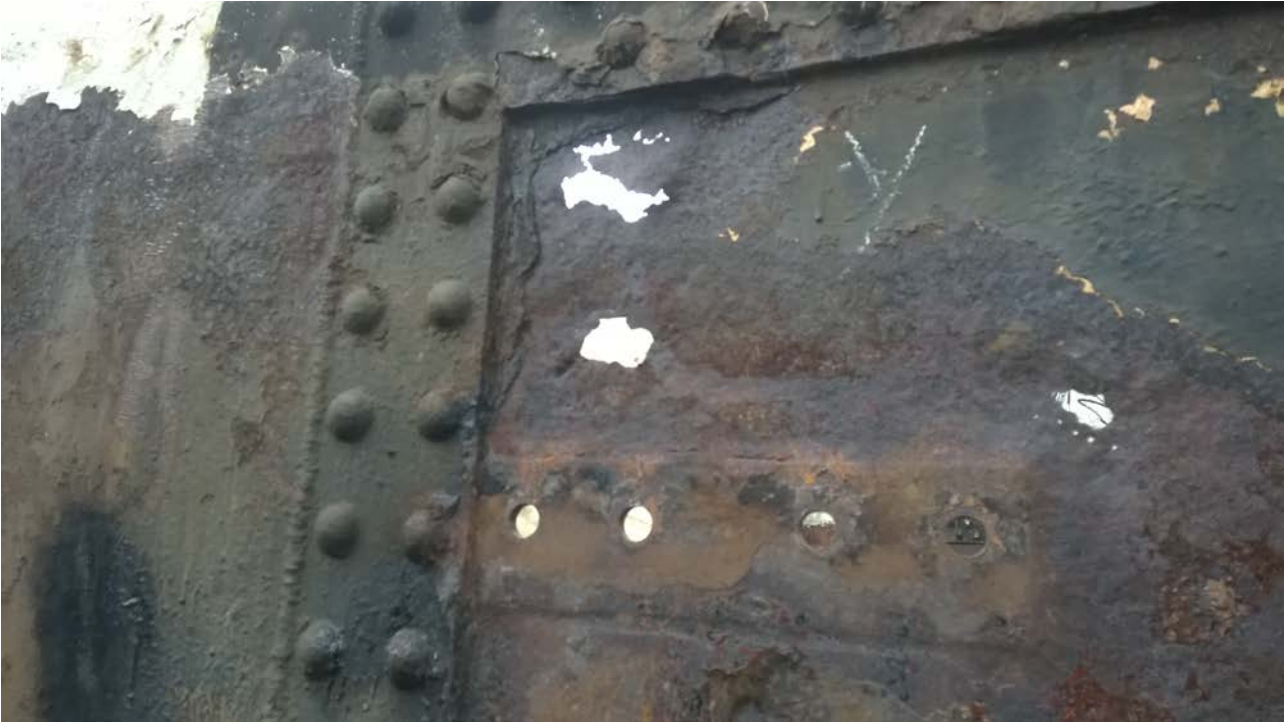
Photo 3 - Perforated main girder web
