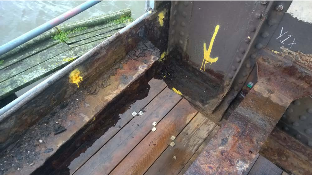
Photo 4 - Missing material on end termination beam flange
