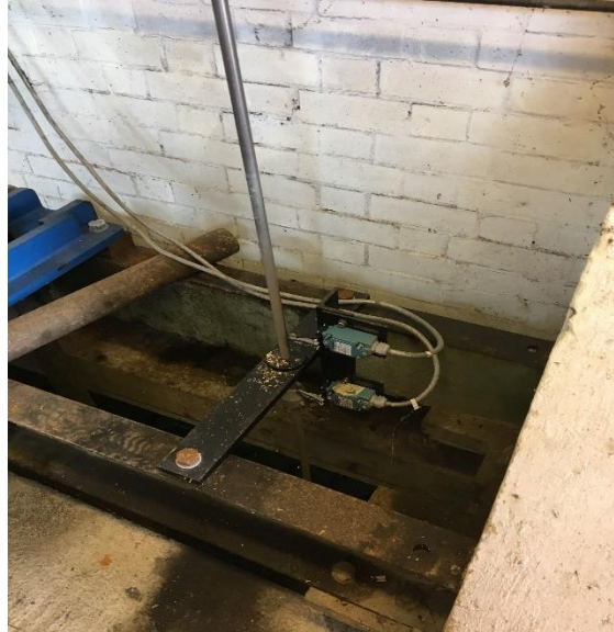
Figure 46: Limit switch cabling
