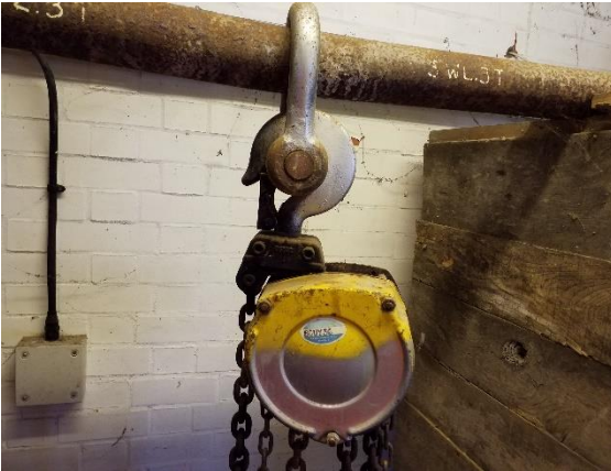
Figure 22: Chain block – emergency plate three
