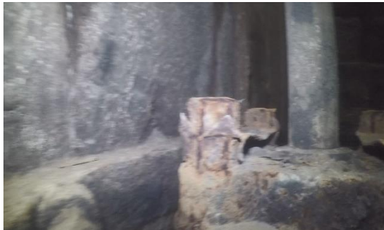
Figure 17: Actuator shaft base - main sluice gate f4
