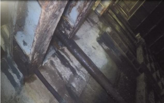
Figure 4: Corrosion on actuator rising stem - main sluice gate 1
