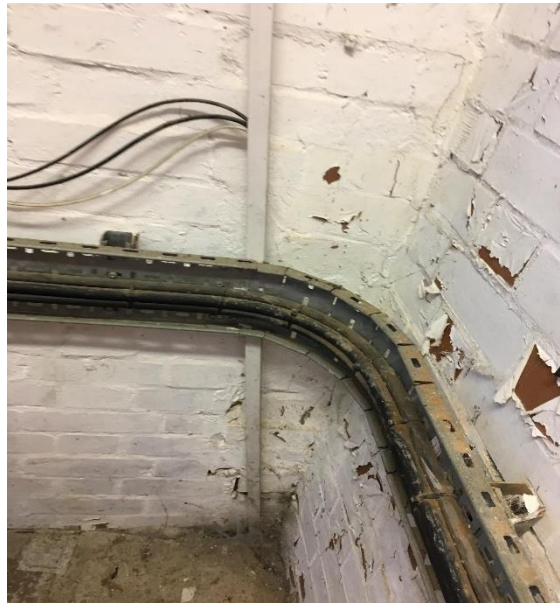
Figure 48: Unsupported cable trunking
