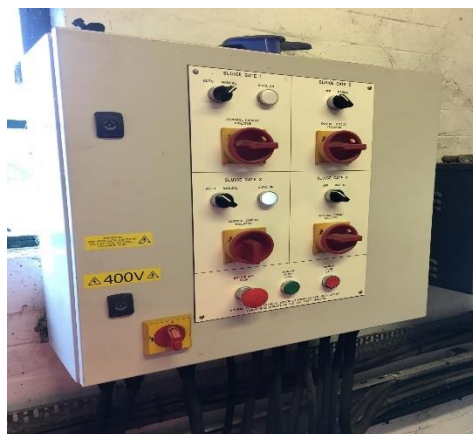
Figure 40: Emergency sluices control panel
