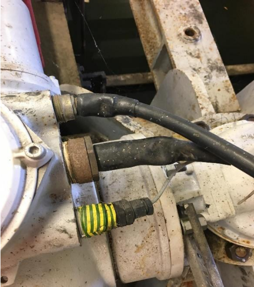
Figure 36: Actuator No.2 cable glands
