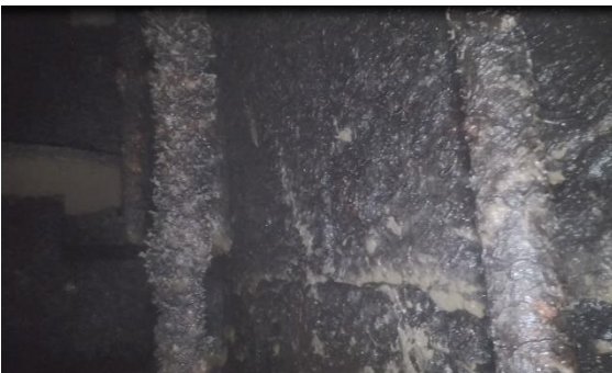
Figure 12: Corrosion on redundant poles– main sluice gate 3
