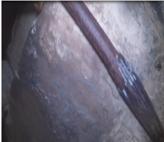
Figure 10: Corroded pole – main sluice gate 2
