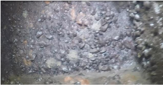
Figure 7: Corrosion and zebra mussels – main sluice gate 2
