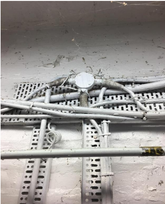
Figure 38: Painted cables and earthing lugs
