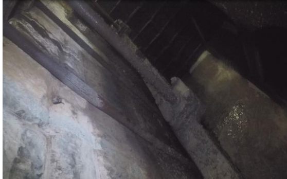
Figure 5: Zebra mussels and corrosion on actuator rising stem base - main sluice gate 1
