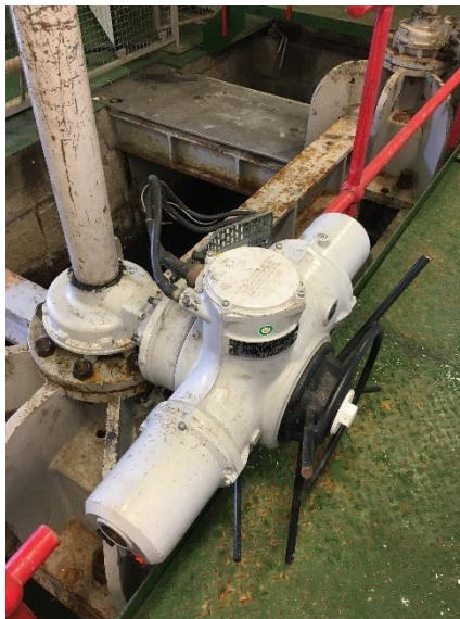
Figure 19: Actuator two – main sluice gate two
