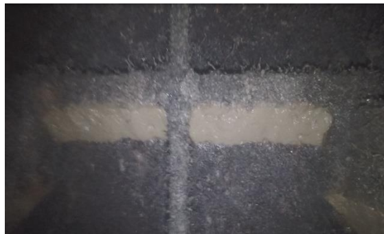
Figure 13: Siltation on gate – main sluice gate 3
