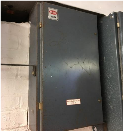
Figure 32: Corrosion on electrical distribution panels
