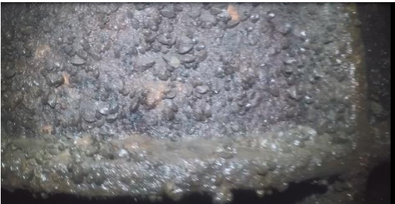
Figure 6: Corrosion and zebra mussels - main sluice gate 1
