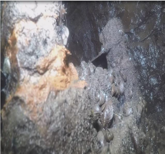
Figure 11 Corrosion at base of rising stem – main sluice gate 2
