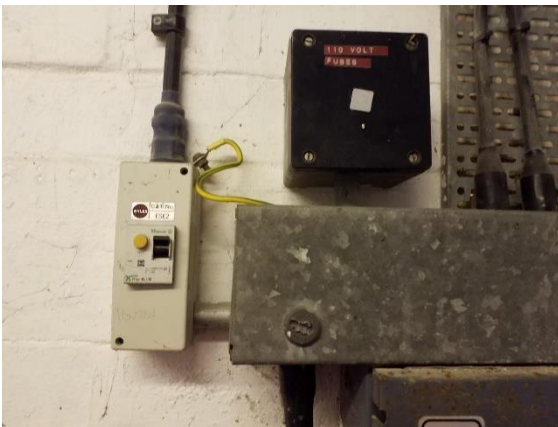
Figure 49: Broken earthing lug
