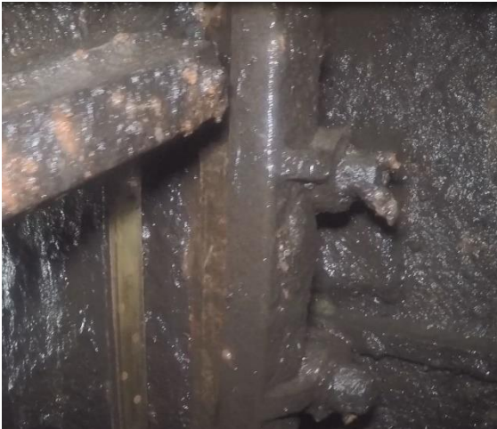
Figure 9: Corroded gate and guide – main sluice gate 2
