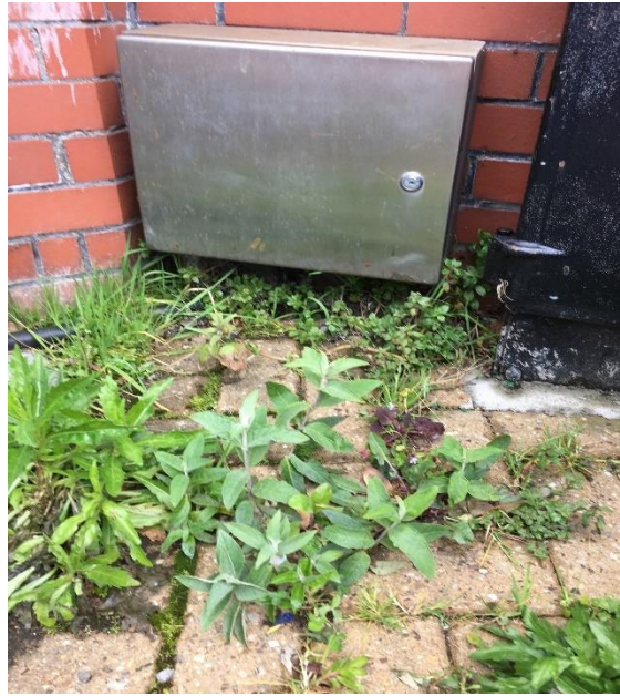
Figure 27: Harbour's level instrument panel
