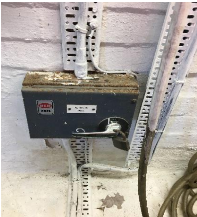
Figure 34: Corrosion on actuators isolators
