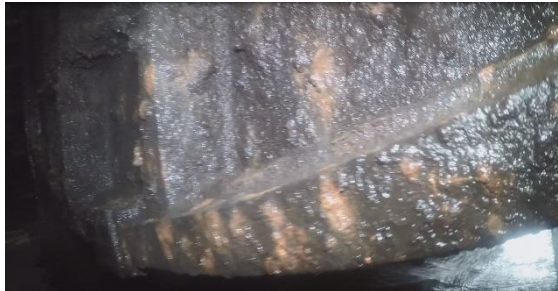
Figure 8: Moderate corrosion on the bottom flange - main sluice gate 2
