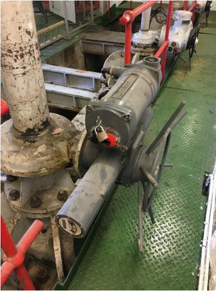
Figure 20: Actuator three – main sluice gate three
