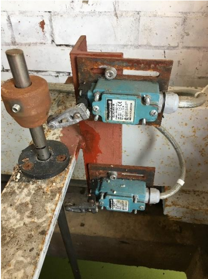
Figure 45: Corroded Limit switch bracket
