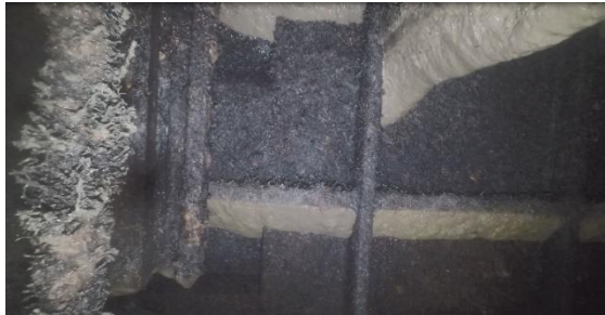
Figure 15: Corrosion on guides– main sluice gate 3
