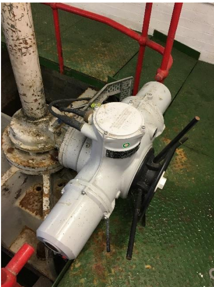
Figure 18: Actuator one – main sluice gate one
