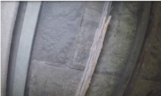
Figure 16: Severely corroded pole – main sluice gate four
