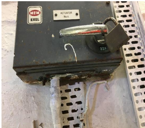
Figure 35: Corrosion on actuators isolators
