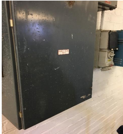
Figure 33: Corrosion on electrical distribution panels
