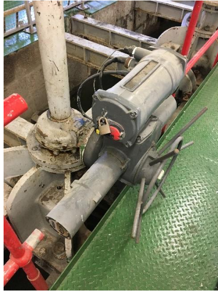
Figure 21: Actuator four – main sluice gate four
