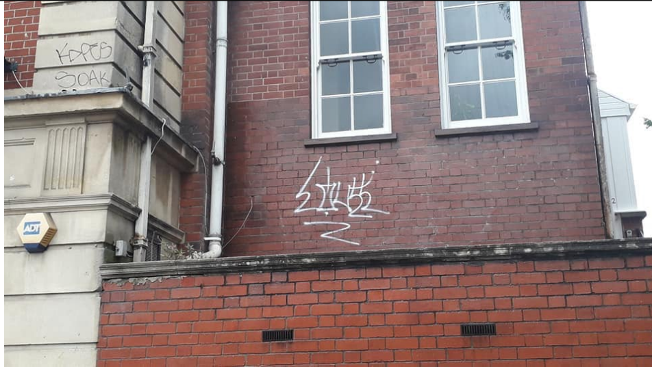
Example 2 of the effectiveness of an AGC coating – 2 Zetland Road – After cleaning
