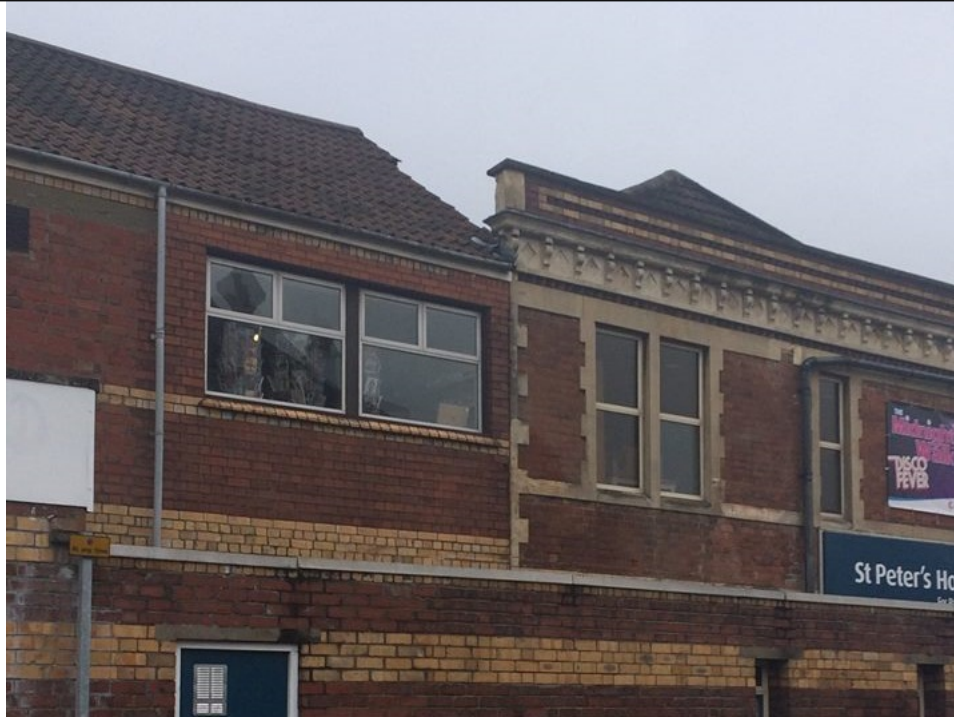
Example 2 of the effectiveness of an AGC coating – 2 Zetland Road - Before
