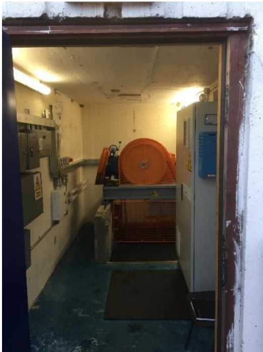
Figure 5-7 Lift motor room Room in good condition with no obvious sources of water ingress
