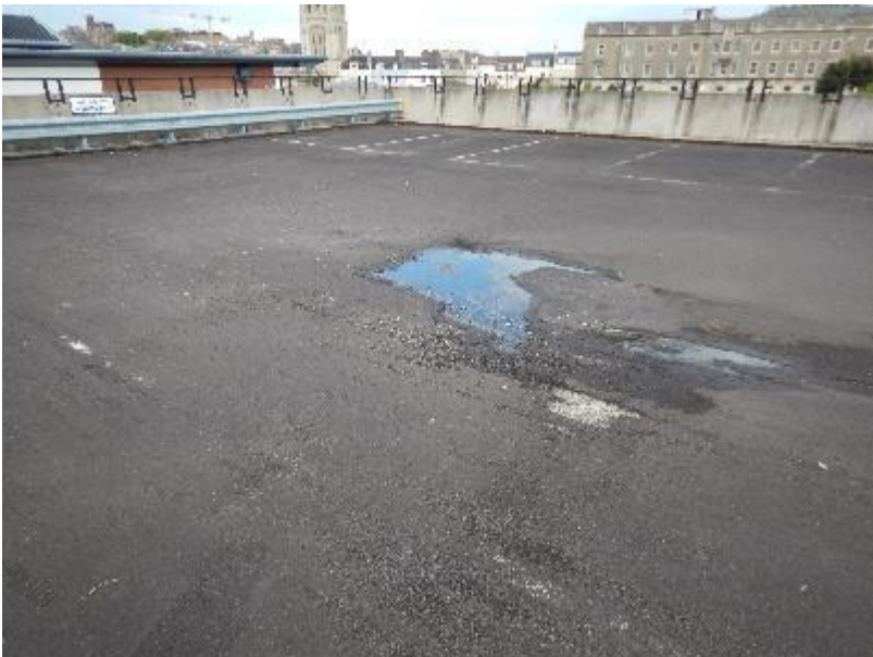
Figure 5-7. Northeast corner of the car park, Level 7B Worn area of bituminous surfacing material
