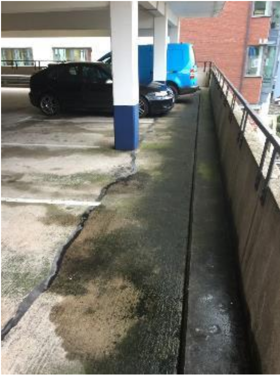
Figure 5-6. Southeast side of the car park looking toward the east corner of the car park Note continuous crack in deck spanning between columns, sealed with bituminous material
