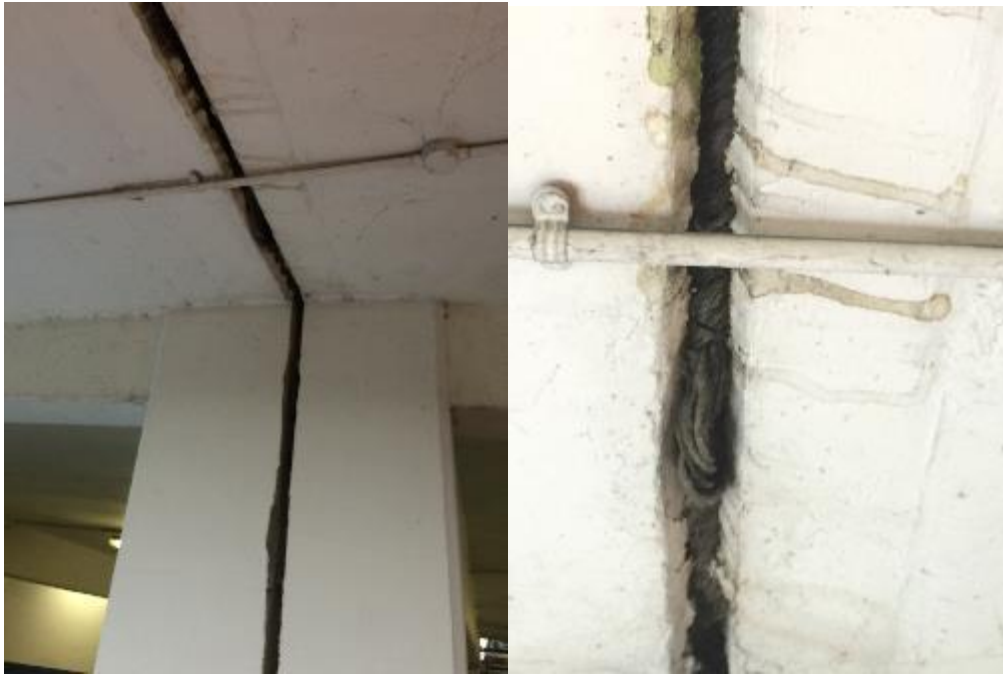
Figure 5-9a (left) and 9b (right). Expansion joint at columns and soffit, intermediate level Note mastic-like sealant between the columns and rope-like infill to the soffit joint.
