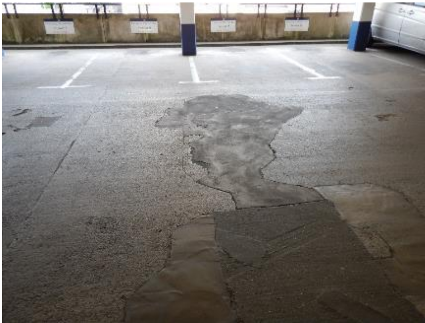
Figure 5-5. Spalling to lower level deck
