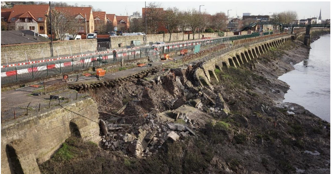
Figure 24: Photo showing the collapse of the riparian wall on Cumberland Road in 2019
