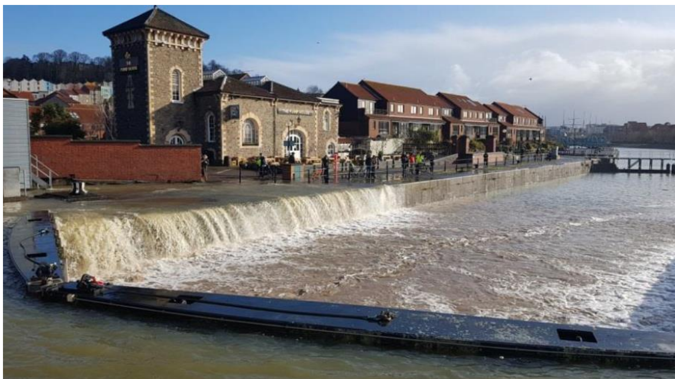
Figure 38: Overtopping at Junction Lock during March 2020 tidal surge
