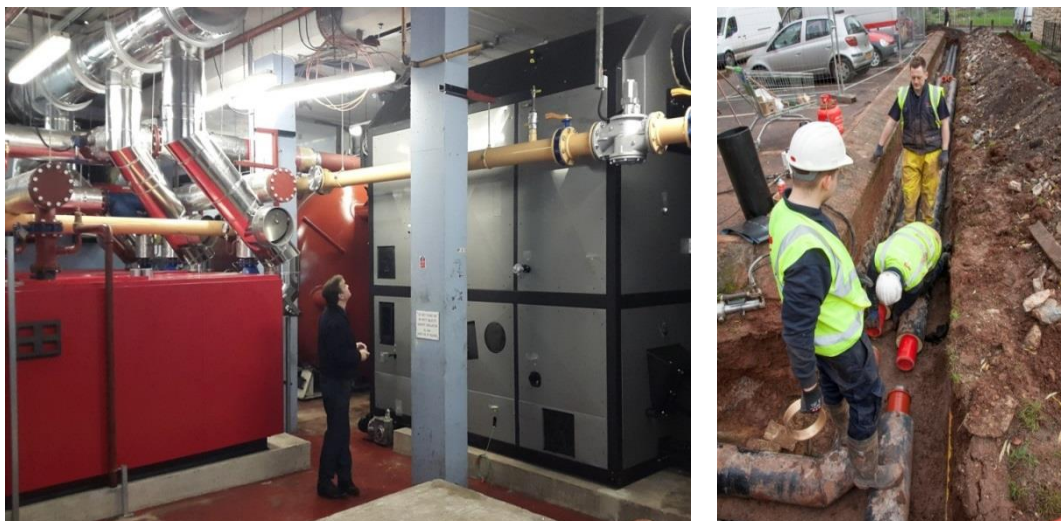
Figure 4: Biomass energy Centre Broughton House and Laying of Rehau PEX pipe as part of Redcliffe Phase 1:
