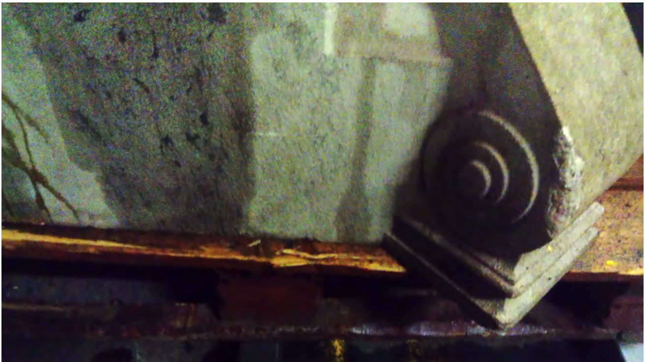
Damaged corner and edges of the stone with significant staining.
